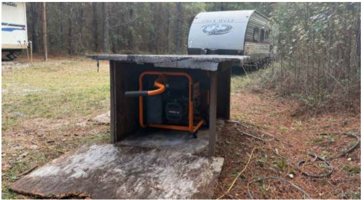
PHOTO # 23: View of a generator in the hunting camp on the northern interior portion of the subject site. View facing southeast.
